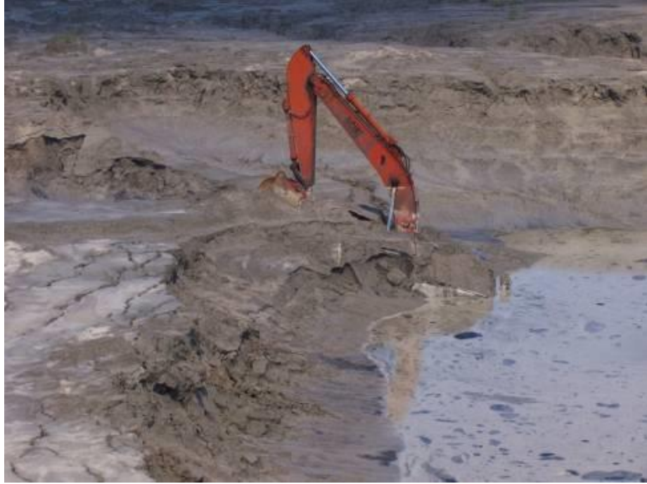
Figure 1.16: Side picture of Trackhoe covered with fly ash caused by fly ash failure at the DPL impoundment
