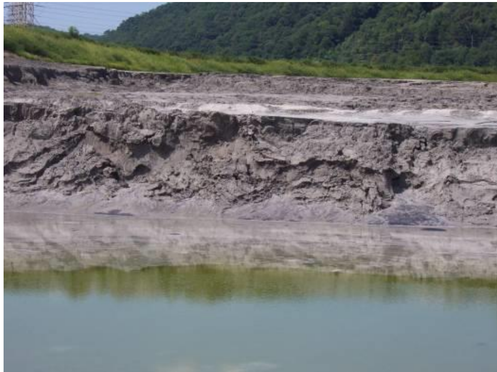
Figure 4.10: Height of impoundment facilities failure at a power plant in Ohio
