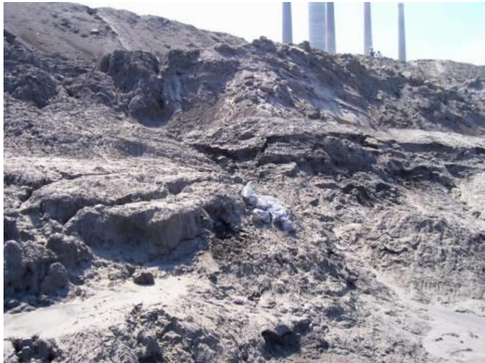
Figure 1.13: Slope failure occurred as a result of fly ash flow at the DPL Power Plant
