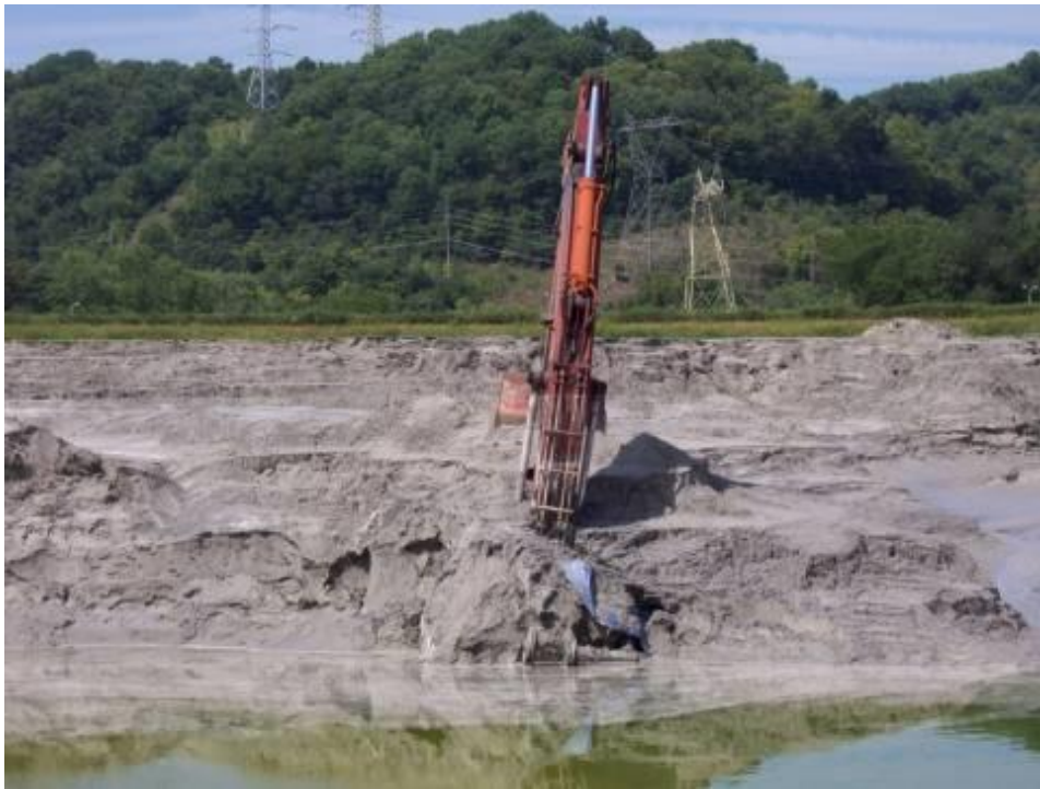
Figure 1.15: Trackhoe engulfed in fly ash at the DPL impoundment after a fly ash failure caused by liquefaction
