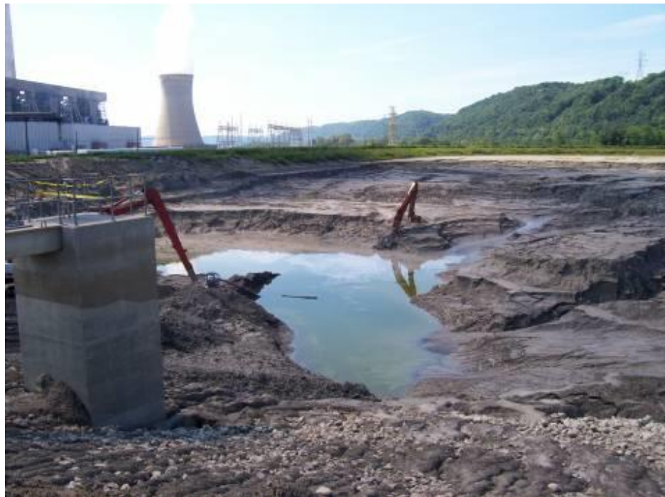
Figure 1.17: Portion of a fly ash flow failure in an impoundment at the DPL power plant
